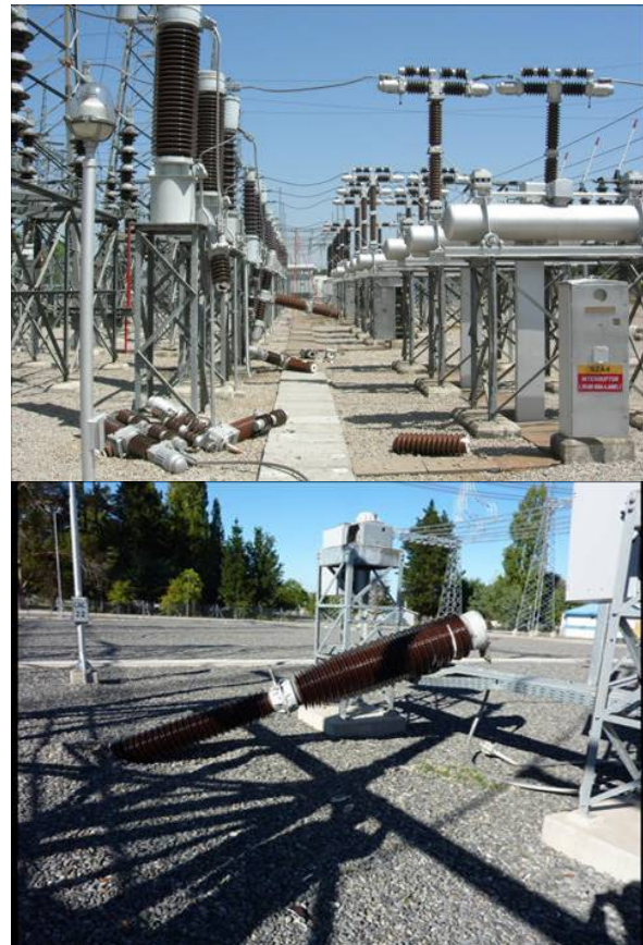
Figure 6.- Transmission equipment damage (Transelec)
